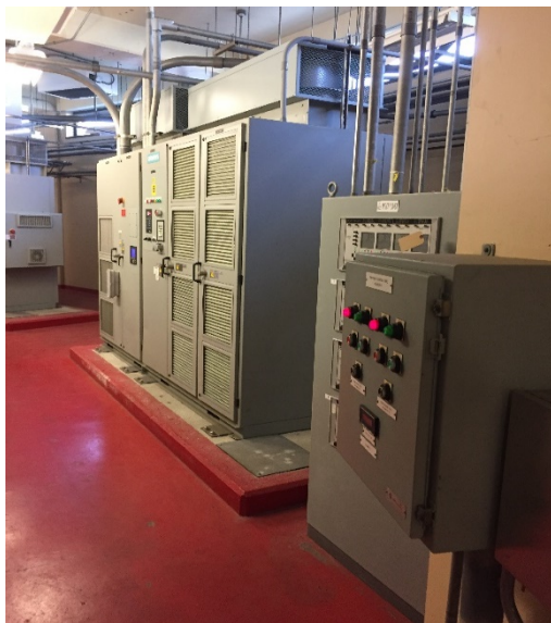
SSPS Pump Variable Frequency Drive
