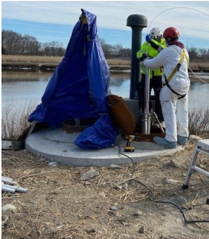
Neponset River Internal Leak Detection Equipment (Hydrophone)
